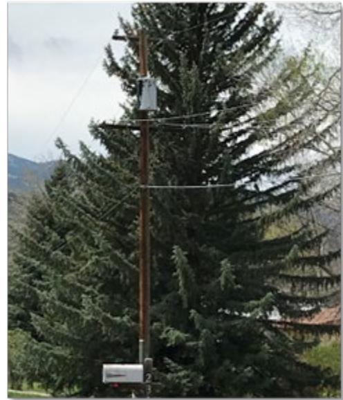
Powerline of Teft Overhead Conversion
