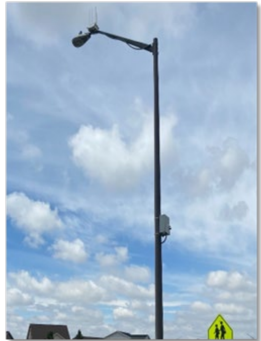
Install of a Gatekeeper and wireless router mounted on a streetlight.
