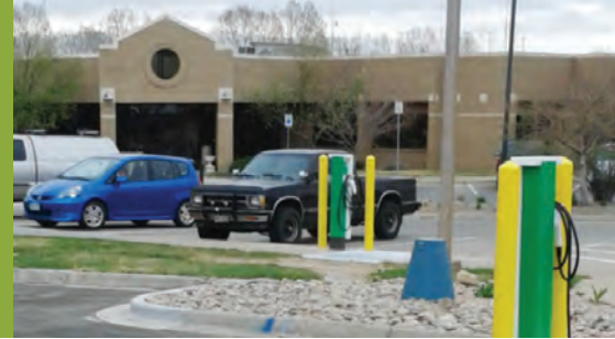
Electric vehicle charging stations
